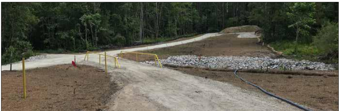
Pictured is a completed passive, in situ groundwater treatment system installed at the Stoller Site in Charleston County.
