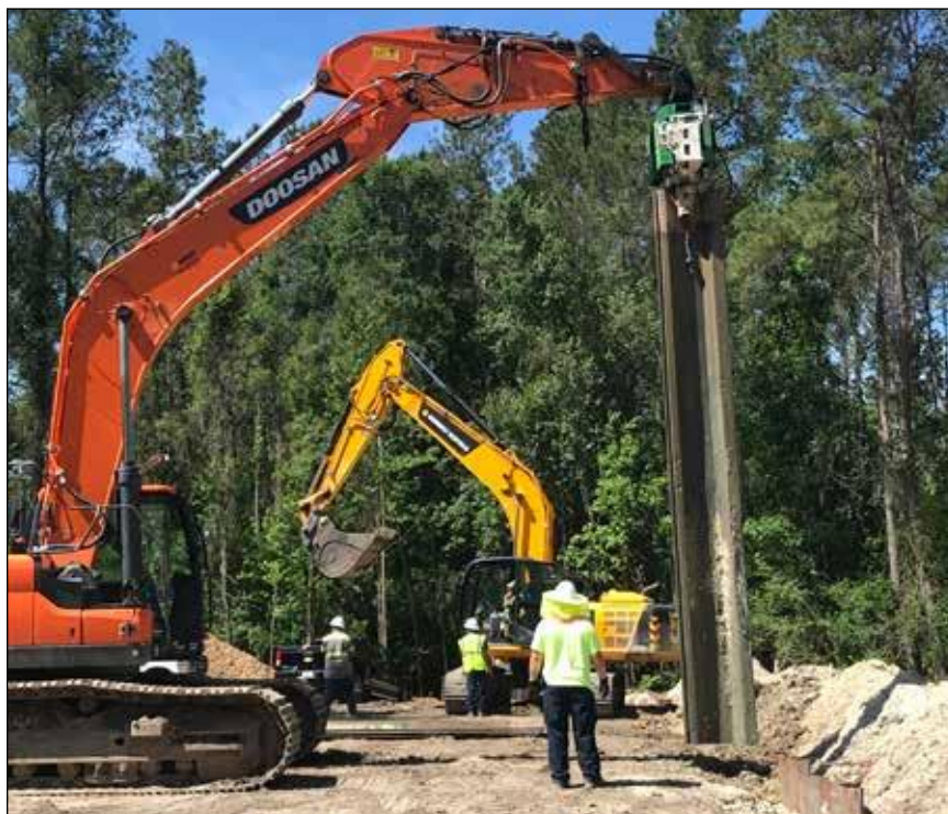
DHEC contractors install the passive, in situ groundwater treatment system at the Stoller Site in Charleston County.
